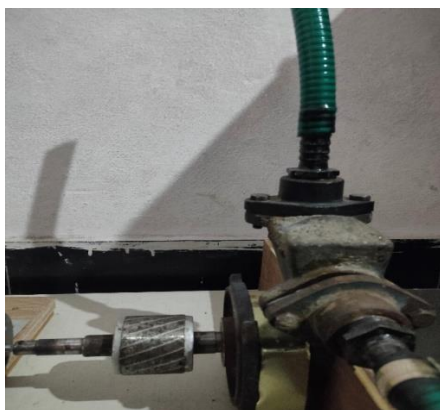
Fig-9: Motor and pump setup
